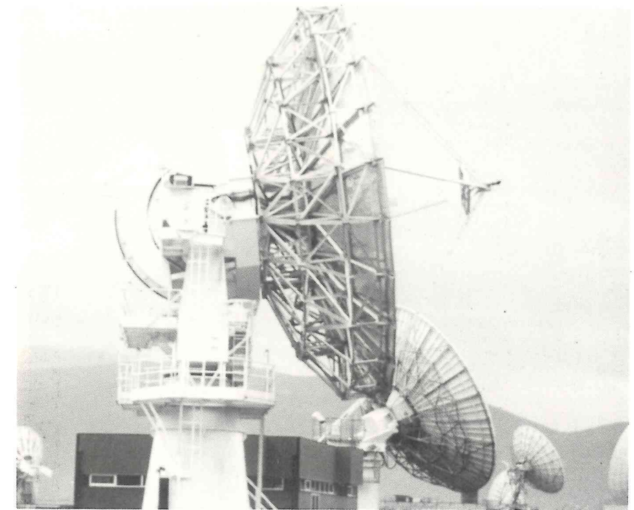
Fig. 93. CES parabolic antenna, Fucino, Italy, (courtesy INMARSAT)
