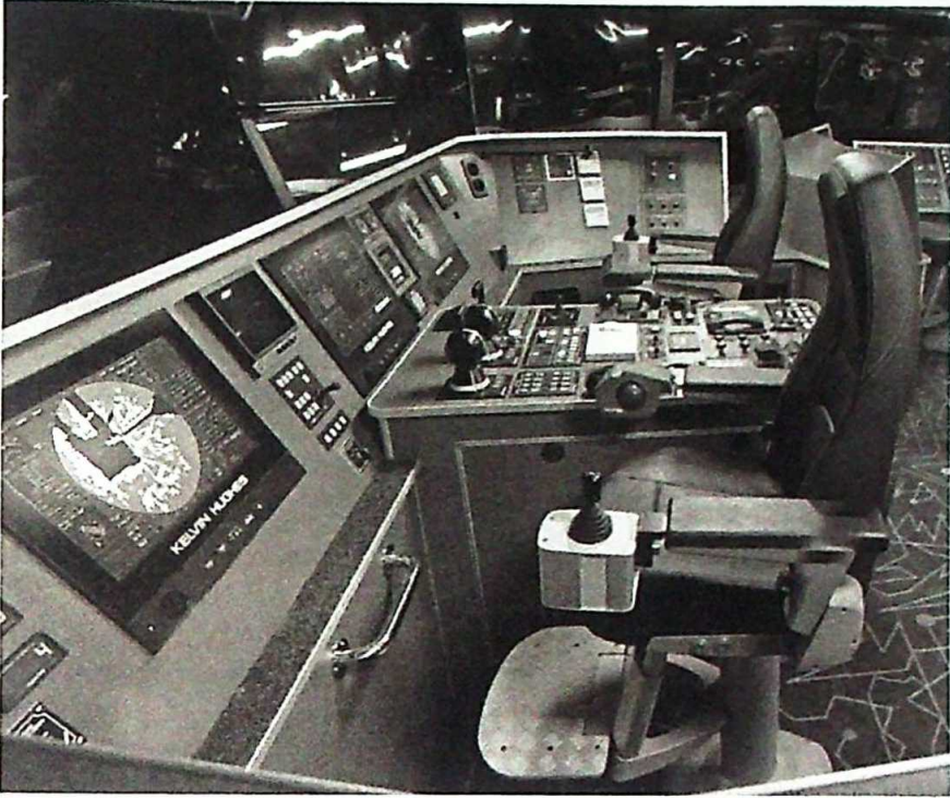
▲ Figure 2.54 Integrated bridge: SharpEye Radar plus ECDIS. Reproduced by kind permission of Austal
