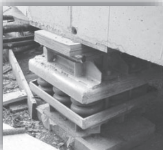
Fig. 8 Springs – with damper base isolator [10]
