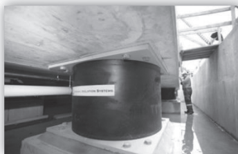
Fig. 7 Lead – rubber bearing in use [10]
