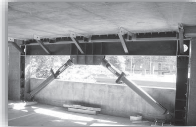
Fig. 11 Viscous damper in use (Aesthetically unpleasing look is evident here) [2]
